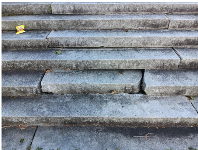
Cracked and loose treads
