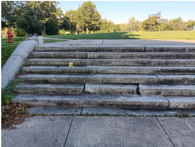
South stairs – cracked and loose treads
