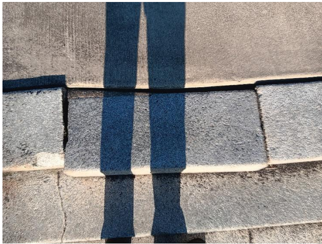
Example - cracked tread, completely loose stairs
