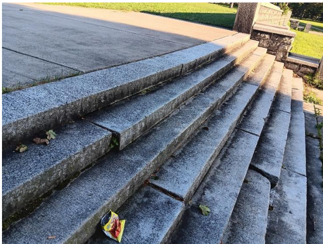
South stairs – lacking joint connections
