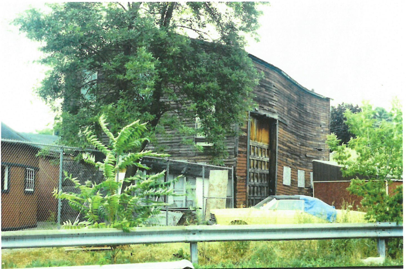
High Bay – Storage Building just before it collapsed in 1995.
