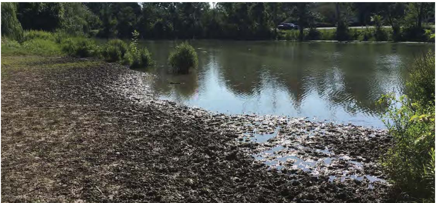
Shoreline conditions need to be addressed on Ellicott Island Bark Park
