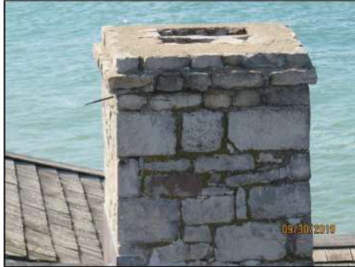
Chimney #7 East side, organic growth, mortar loss, iron embedment
