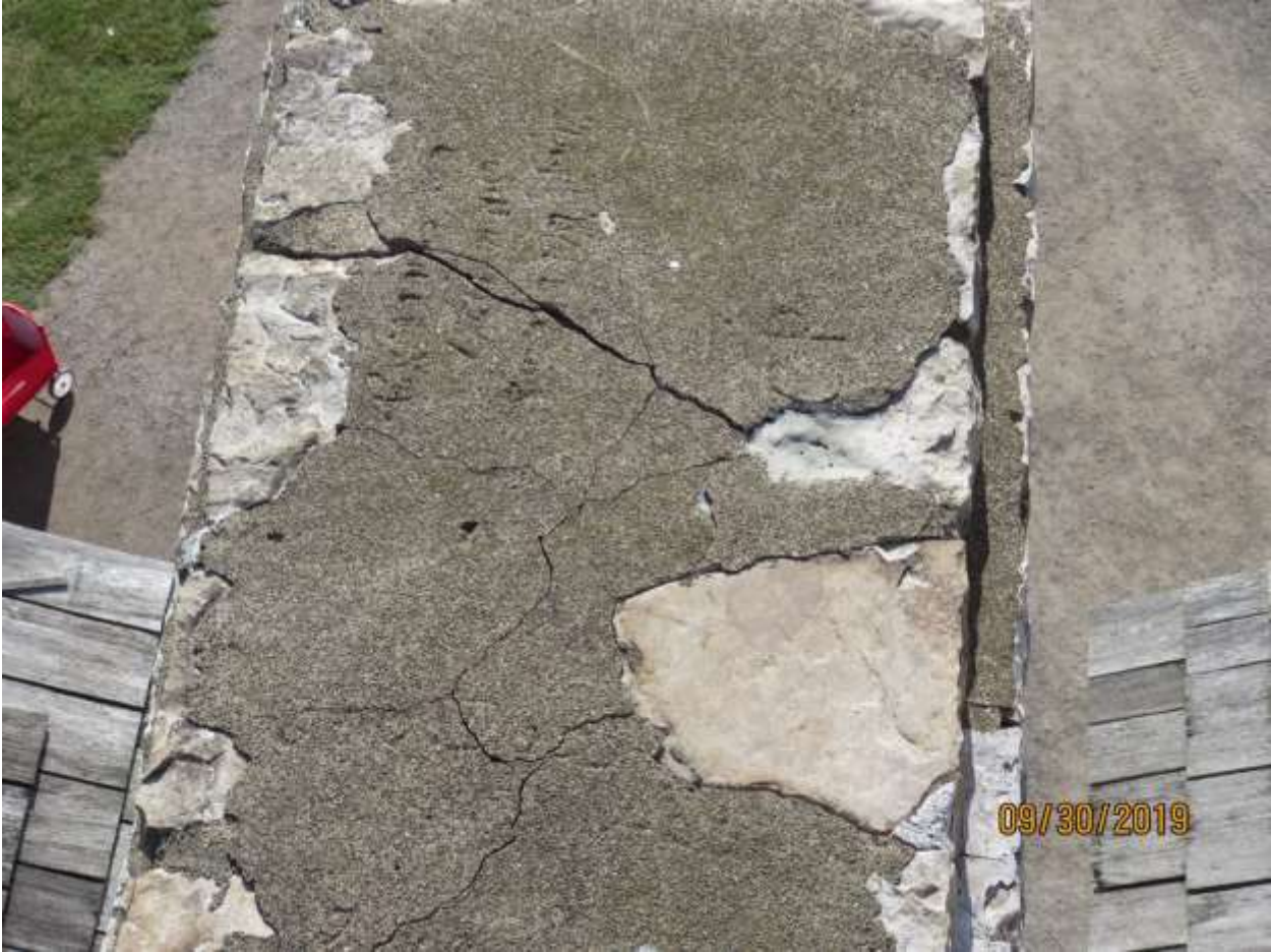
E2 - Chimney #4 cracked parging / open joints at cap
