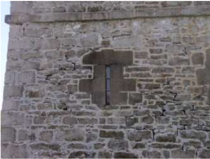
Detail C — 14' x 10.5' area of masonry showing two large areas of mortar loss totaling about 10 square feet, plus other smaller losses.
