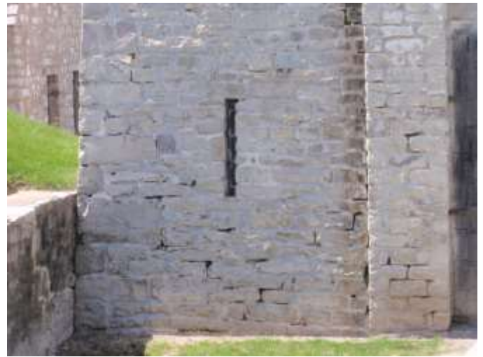
Detail A — 13' x 10.75' area of masonry showing several small areas of mortar loss totaling approximately 30 linear feet.
