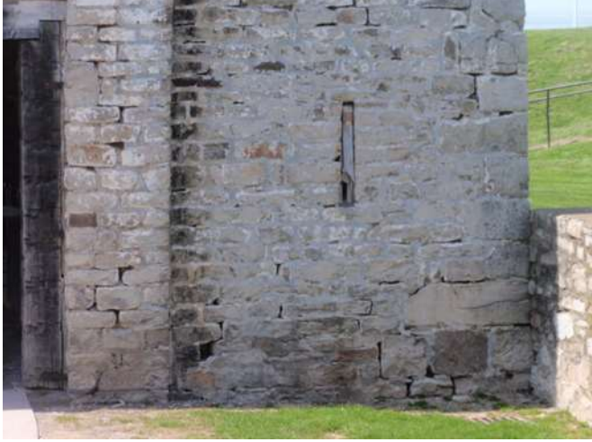
Detail F — 13' x 10.75' area of masonry showing numerous small areas of mortar loss totaling approximately 40 linear feet.
