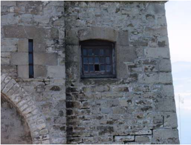
Detail E — 13.5' x 11' area of masonry showing numerous small areas of mortar loss totaling about 13 linear feet.
