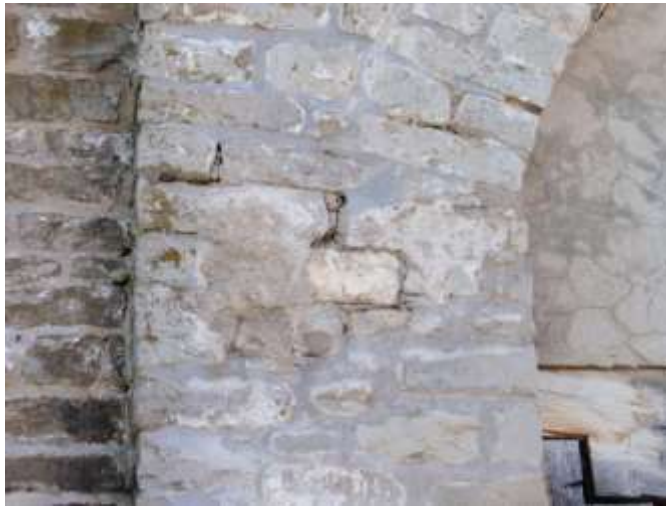
Detail C — 5' x 3.75' area of masonry showing approximately 4 linear feet of mortar losses, plus another partial view of the universally cracked stucco façade lining the arch behind the coat of arms.
