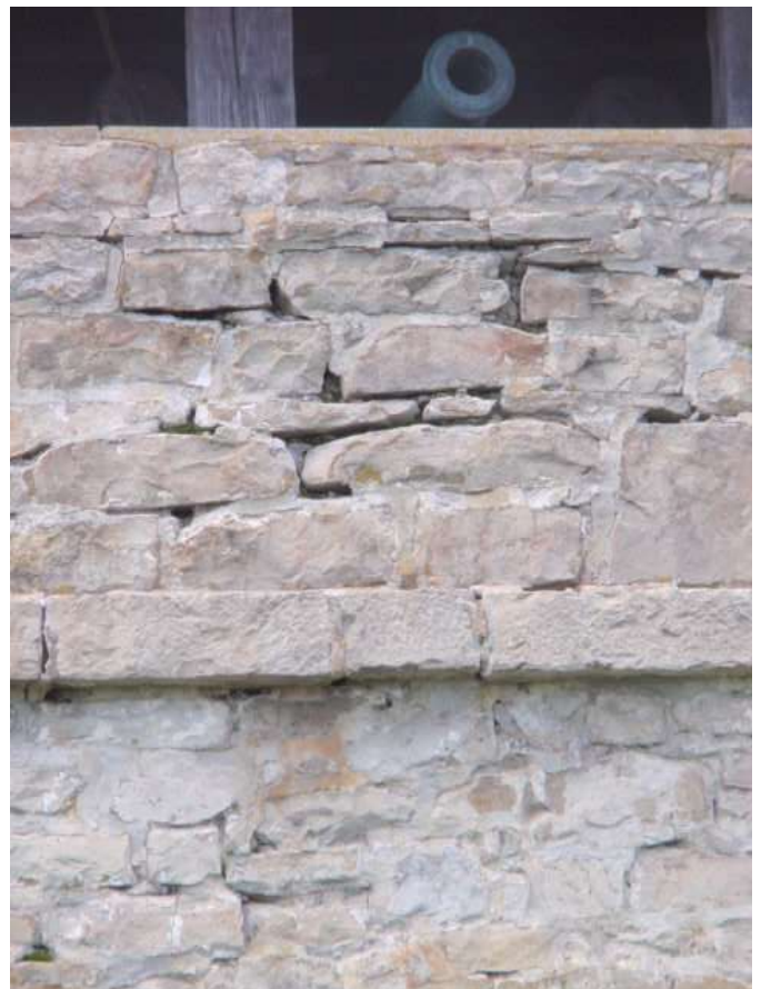
Detail B — 6' x 6.25' area of masonry showing mortar losses totaling approximately 9 linear feet.
