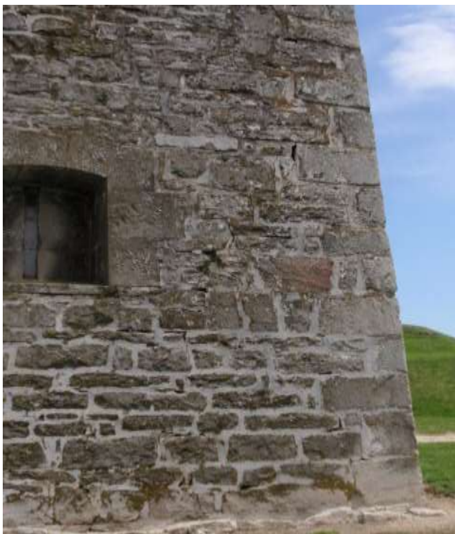
Detail C — 10' x 12' area of masonry showing about a dozen small mortar losses ranging averaging 5" in length, and a rambling vertical crack extending approximately 6.5 linear feet overall.
