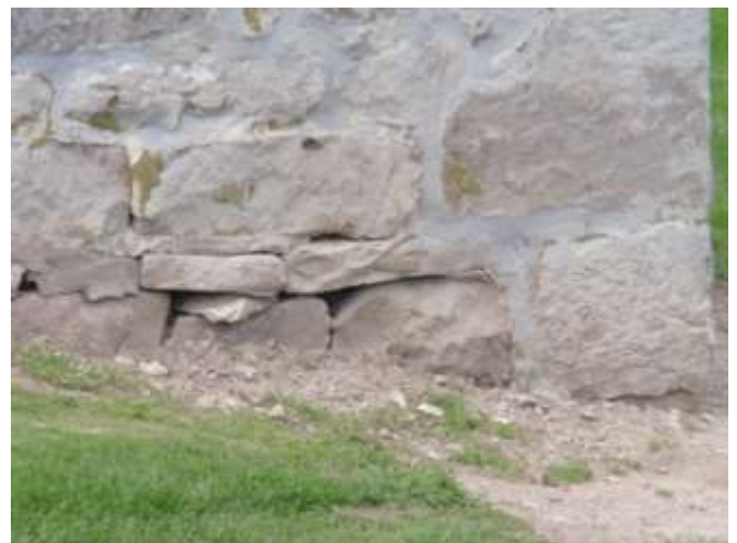
Detail H — 5' x 2.5' area of masonry showing loose stones and mortar losses ranging from 2" to 2' in length.
