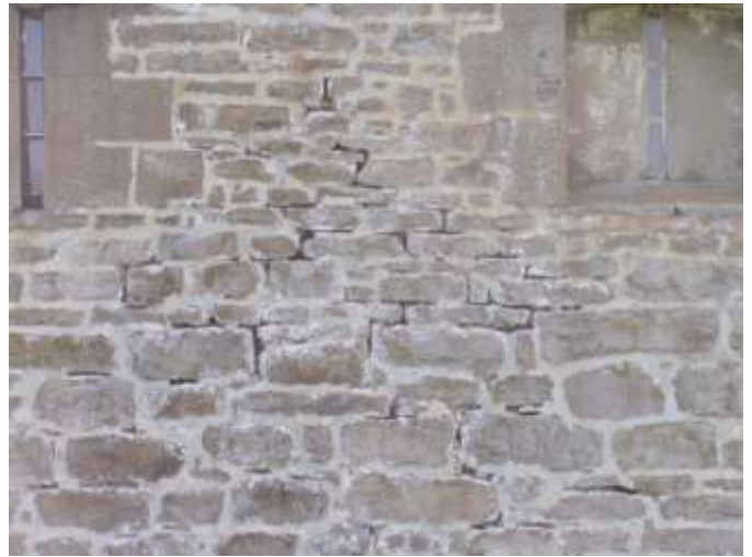
Detail D — 11' x 8.5' area of masonry showing a 28 square foot area of significant mortar loss, plus other smaller losses.
