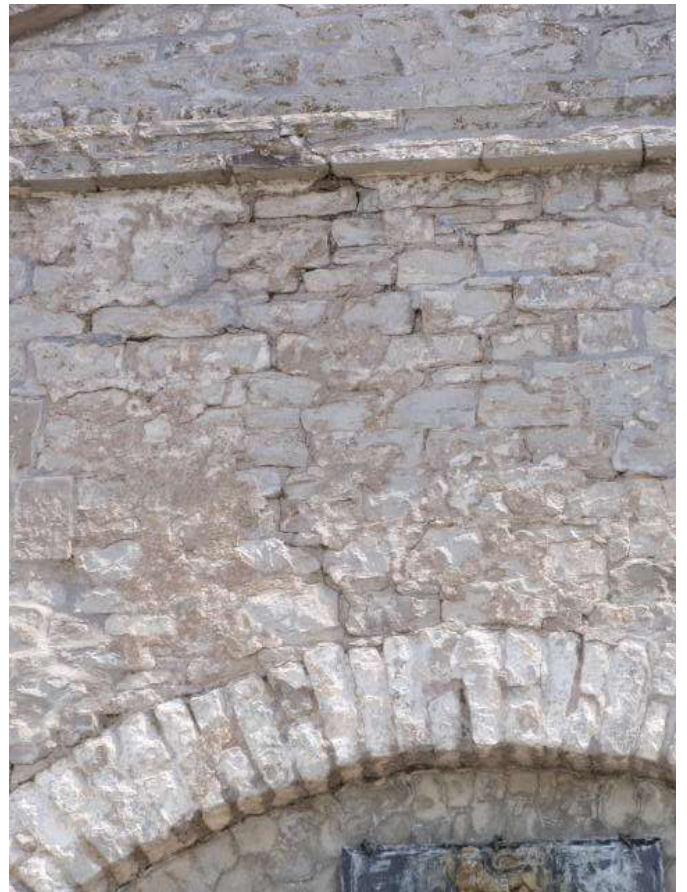
Detail B — 8.5' x 11' area showing a rambling vertical crack extending for approximately 8 linear feet, plus numerous small mortar losses throughout. Note that the stucco façade lining the arch behind the coat of arms is also universally covered with hairline cracks.
