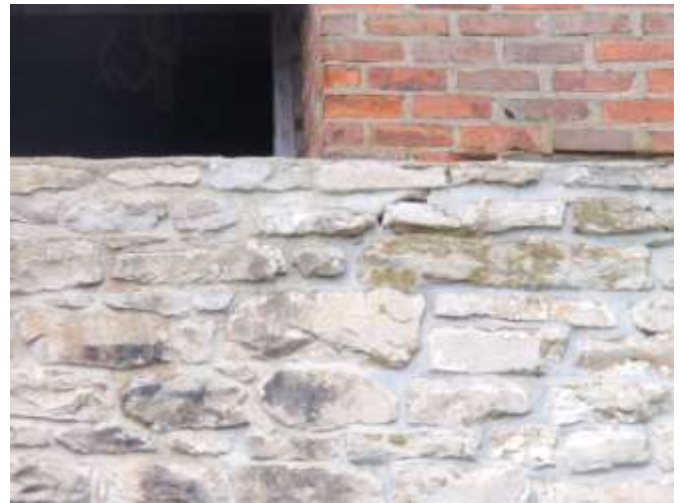
Detail A — 3' x 5' area of stone masonry showing mortar losses totaling about 2 linear feet, plus a 4 square foot area probably repointed in 1987.
