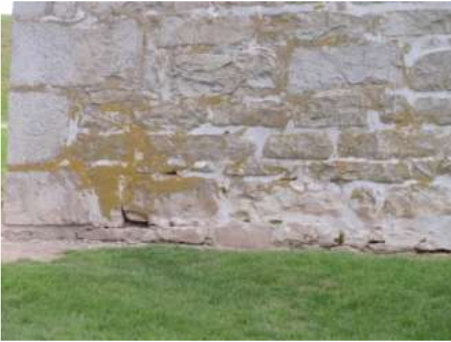
Detail C — 8.5' x 4.75' area of masonry showing mortar losses along the building's foundation ranging in length from 4" to 8".
