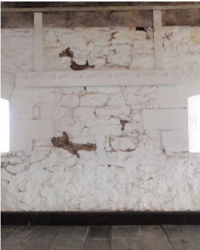
Detail F — 6.5' x 6' area of masonry showing several prominent, rambling vertical cracks and other areas of loss.
