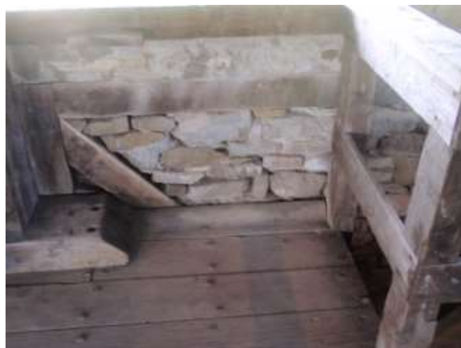
Detail A — 7.5 square foot area of severe mortar loss on covered gun deck.
