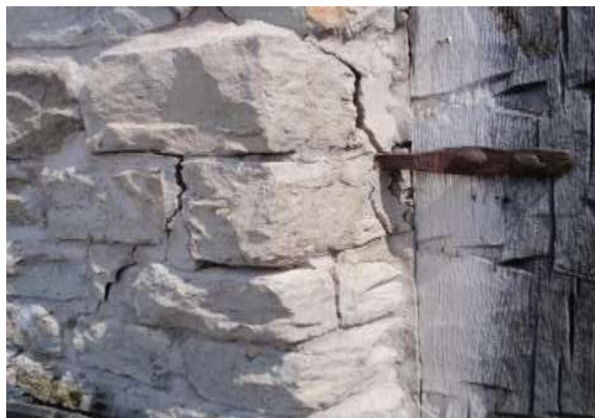
Detail D — 4' x 4' area of masonry showing approximately 14 linear feet of large mortar cracks — and potential for loss of limestone blocks — associated with the iron pintles securing the gateway arch. There are a total of six similar pintles on the South Redoubt's gateway arches. All of them have a similar situation.
