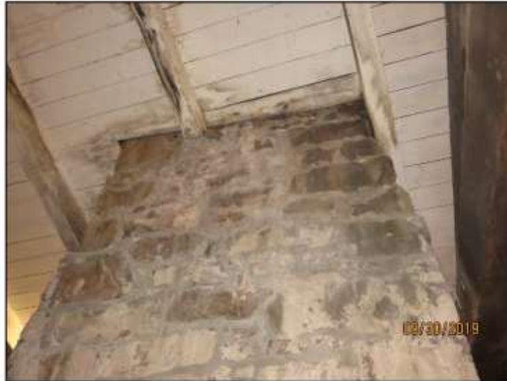
Typical staining from previous leaks - Typical
