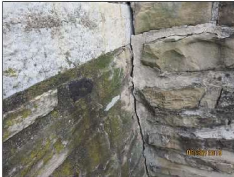
Chimney #2 Close up of Cold joint / separation from building
