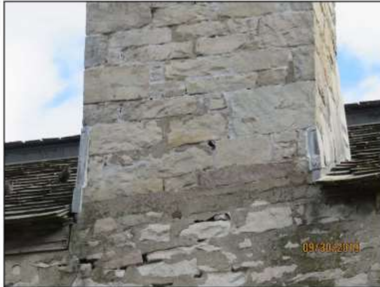
Chimney #6 Mortar Loss – West Side
