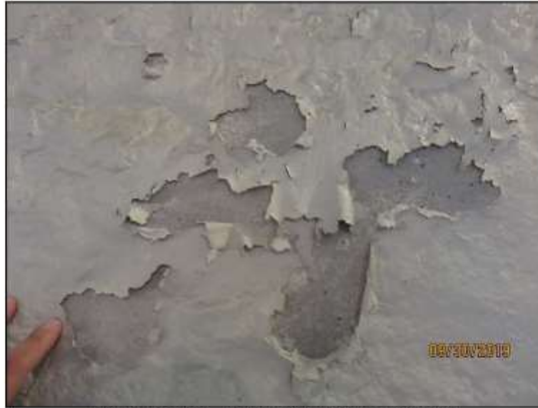
Peeling coatings – Commandant’s Council Chamber
