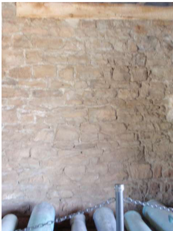
Detail A — 9' x 11'xxx area of masonry showing two rambling areas of cracked and/or lost mortar — one running from top to bottom on the right, and one from the middle of the image to the bottom — together totaling approximately 21 linear feet, in addition to other random small losses.
