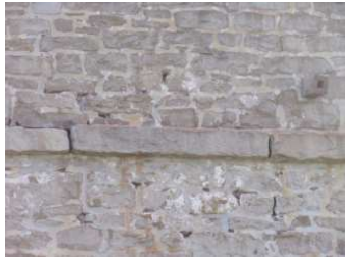
Detail A — 6' x 4.5' area of masonry showing numerous small areas of mortar loss totaling approximately 6.5 linear feet, plus a loss of mortar between the stones of the belt course.
