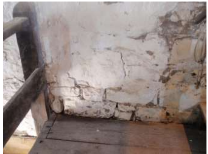
Detail H — 3' x 4' area of masonry numerous instances of lost mortar and/or cleaving stones.
