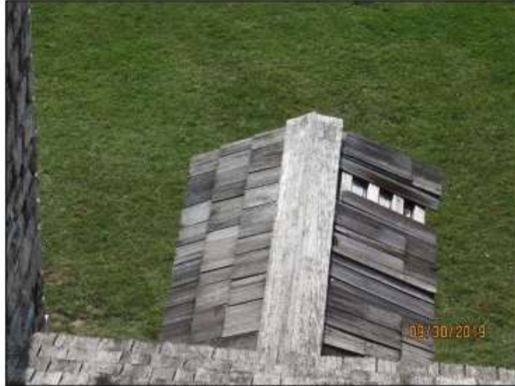
Missing shingles on dormers
