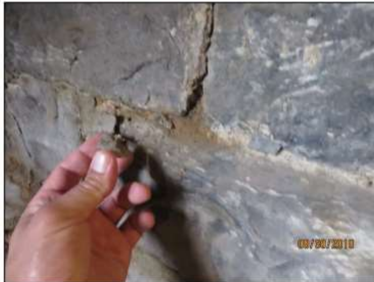
Mortar loss at firebox
