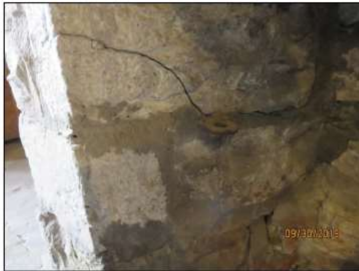
Rusts jacking of pot holder anchor - Typical
