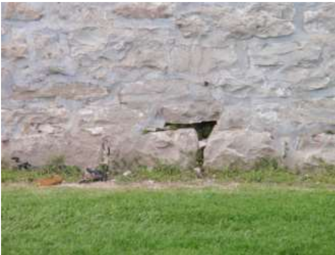
Detail E — 6' x 3.25' area showing about 1 square foot of missing stone and/or mortar along the building's foundation.
