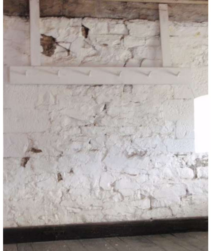
Detail G — 6.5' x 6' area of mortar showing several prominent areas of mortar loss.
