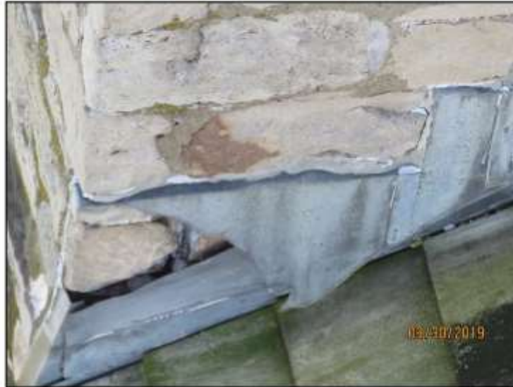
Chimney #2 North Side -Loss of flashing
