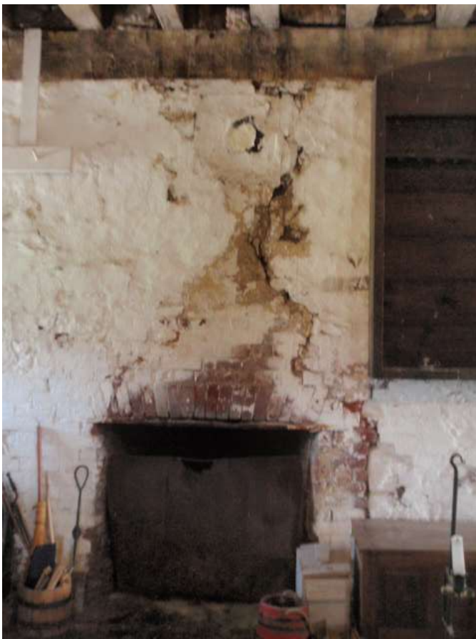
Detail Area A — 8.5' x 10' area of masonry showing a large rambling vertical crack extending from the fireplace to the ceiling, and another long vertical crack to the right of the fireplace.
