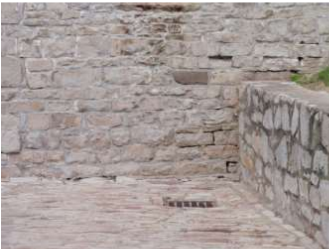
Detail H — 12' x 5.5' the continuation of the crack from Detail G, plus various other small losses totaling approximately 14 linear feet.
