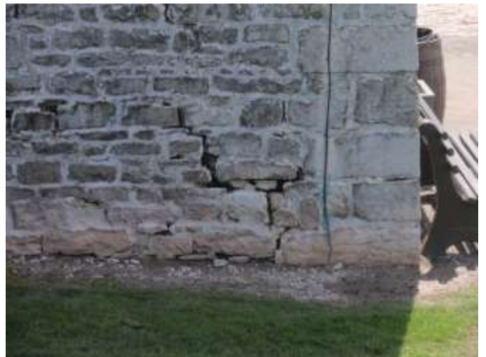
Detail H — 8' x 5' area of masonry showing a closer view of the area in the lower right of Detail G.
