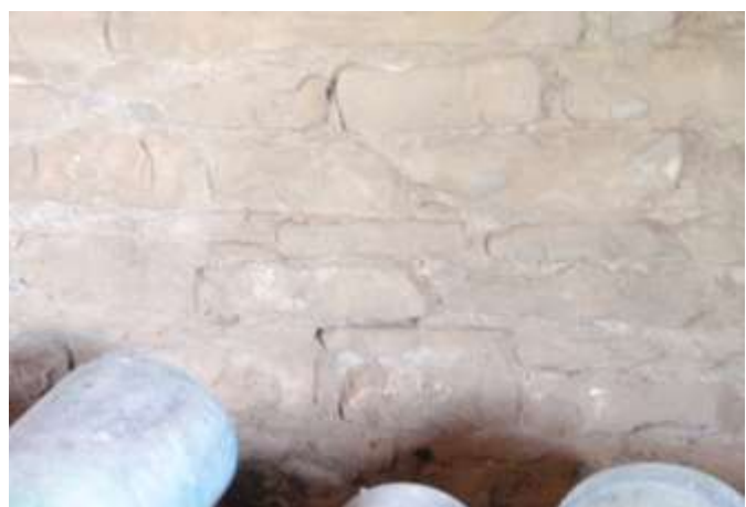
Detail D — Close up of 1.5' x 3' area of masonry at the bottom middle of Detail A.
