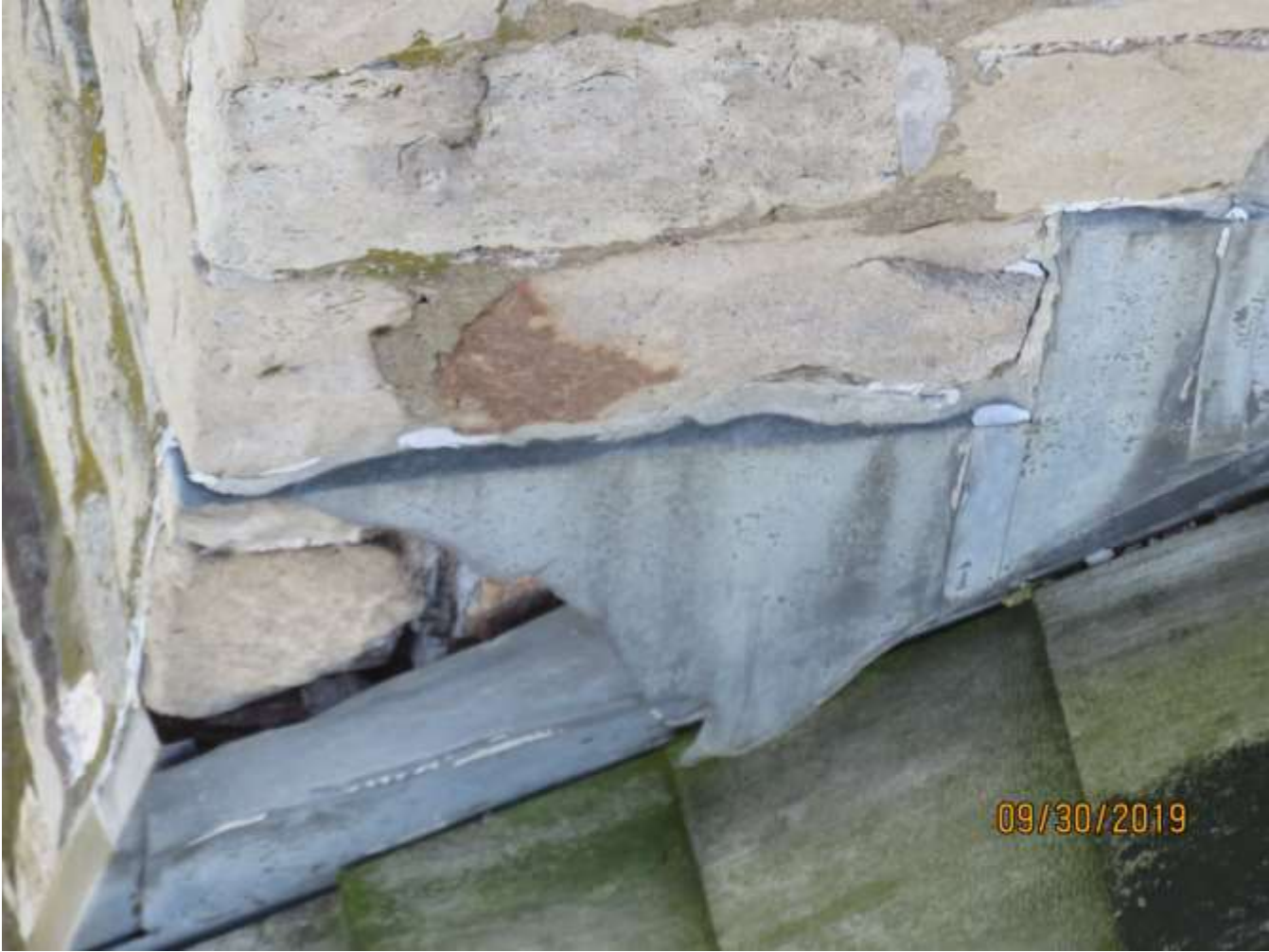
E3 - Chimney #2 North Side -Loss of flashing
