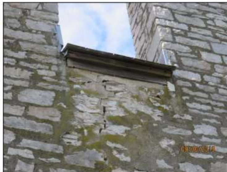
Voids between Chimneys 1&2
