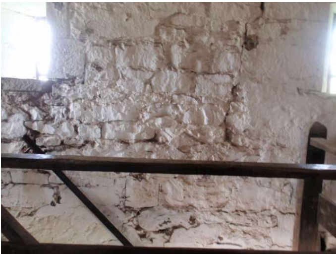
Detail F — Roughly 9' x 6' area of masonry showing significant areas of lost mortar and cleaving stones, plus a partial view a long vertical crack (right, see Detail G).
