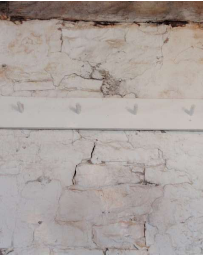
Detail D — 2' x 2.5' area showing a pair of rambling vertical cracks extending approximately 5 linear feet overall plus additional signs of water infiltration.
