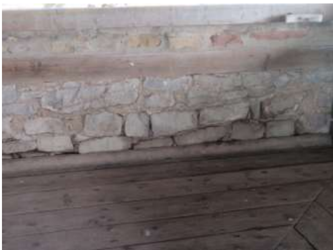
Detail B — 9 square foot area of severe mortar loss on covered gun deck
