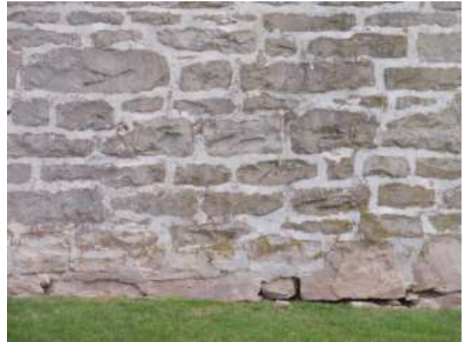
Detail F — 7.5' x 4.75' area showing mortar losses along the building's foundation ranging in length from 3" to 3 linear feet.
