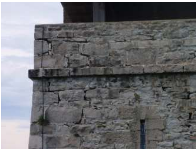
Detail A — 13' x 10' area of masonry showing several rambling mortar losses with a total of approximately 16 linear feet, plus other small areas of loss.
