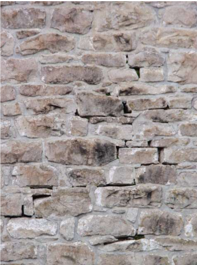
Detail D — 5' x 7' area of masonry showing numerous small areas of mortar loss totaling approximately 13 linear feet.
