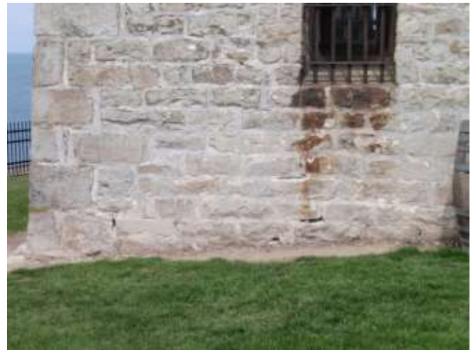
Detail B — 11' x 6' area of masonry showing several small mortar losses ranging from 4" to 10" each.
