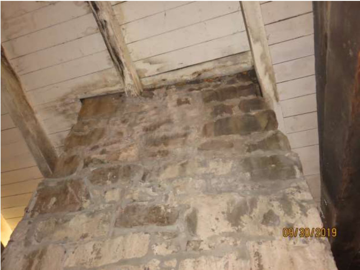
E5 - staining from previous leaks
