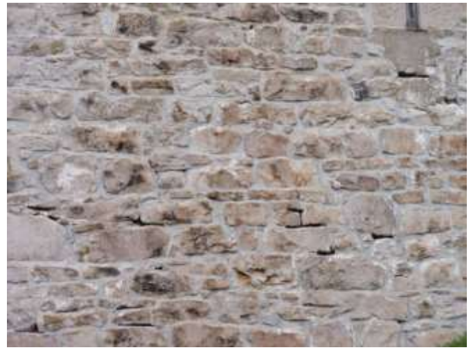
Detail E — 8' x 10' area of masonry showing numerous small areas of mortar loss totaling approximately 9 linear feet.
