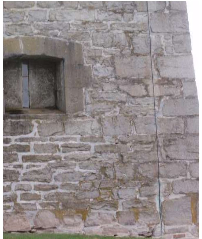
Detail B — 10' x 11.5' area of masonry showing several mortar losses along the building foundation and a rambling vertical crack extending approximately 8 linear feet overall.
