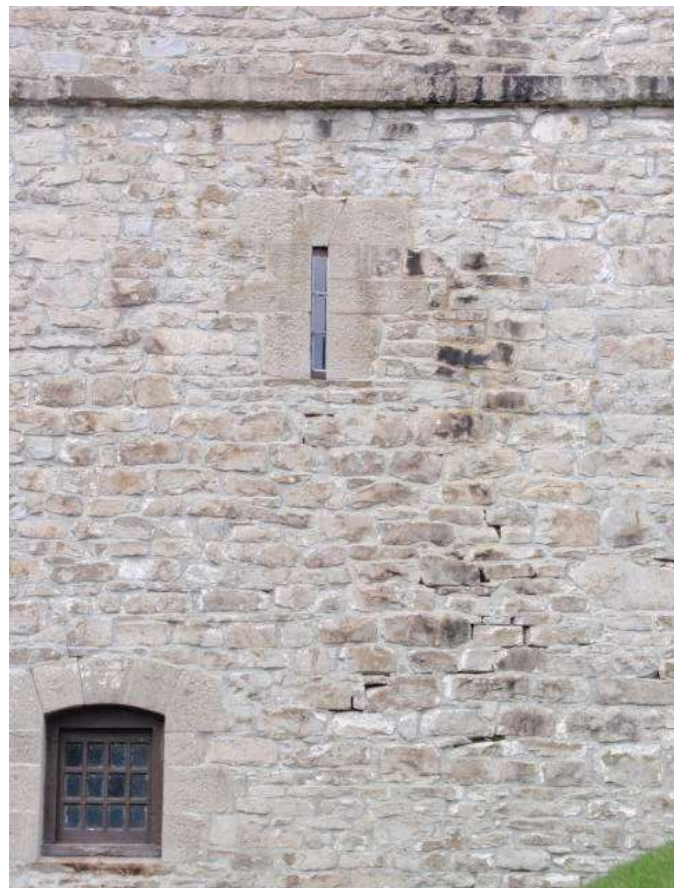
Detail B — 13.5' x 18' area showing numerous small mortar losses totaling approximately 30 linear feet.
