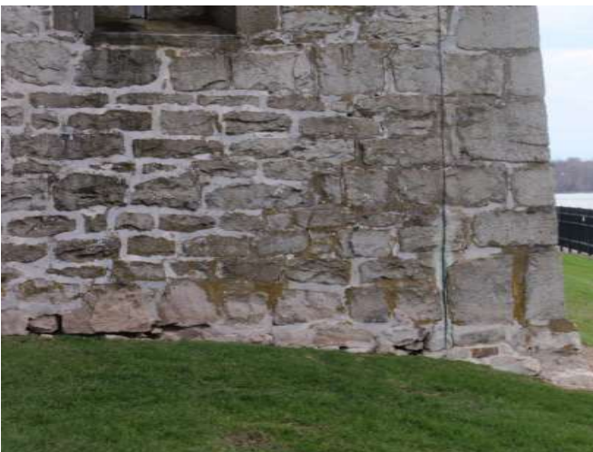
Detail G — 13' x 7.5' area of masonry showing a rambling vertical crack extending approximately 7 linear feet overall, and various mortar losses along the building's foundation ranging from 6" to 3 linear feet.
