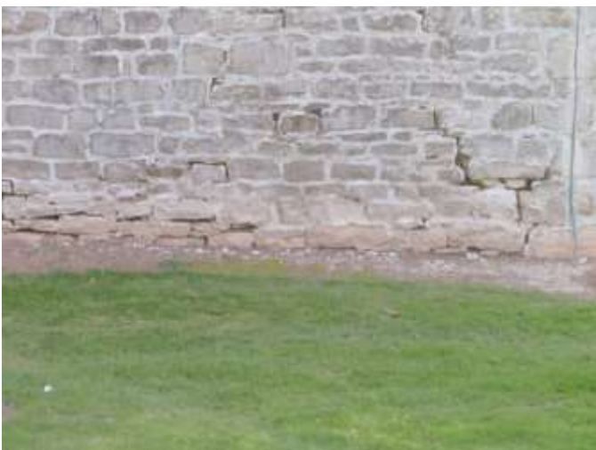
Detail G — 13' x 5.5' area showing a large, rambling area of loss (lower rt) extending 7 linear feet, a 12 sq. ft. area of loss along the foundation (lower left), plus several smaller losses.
