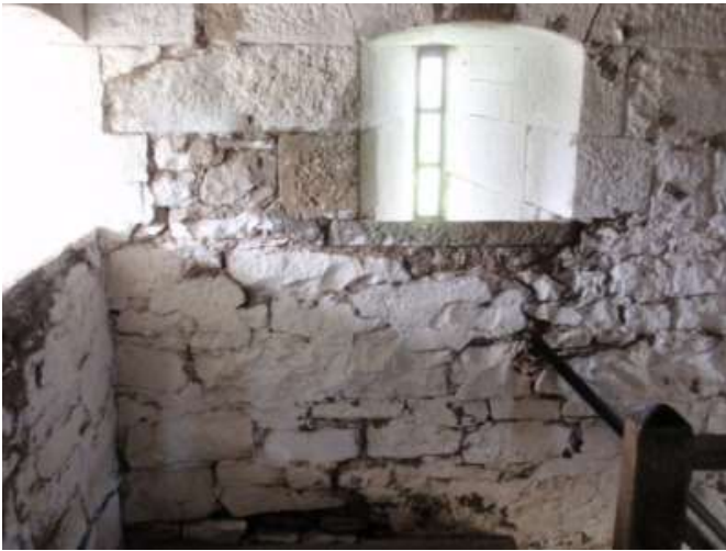
Detail D — 6' x 5' area of masonry showing significant areas of lost mortar and cleaving stones.
