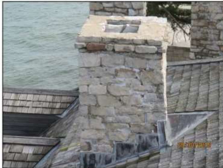
Chimney #8 -Typical Mortar loss and inconsistent composition West Side
