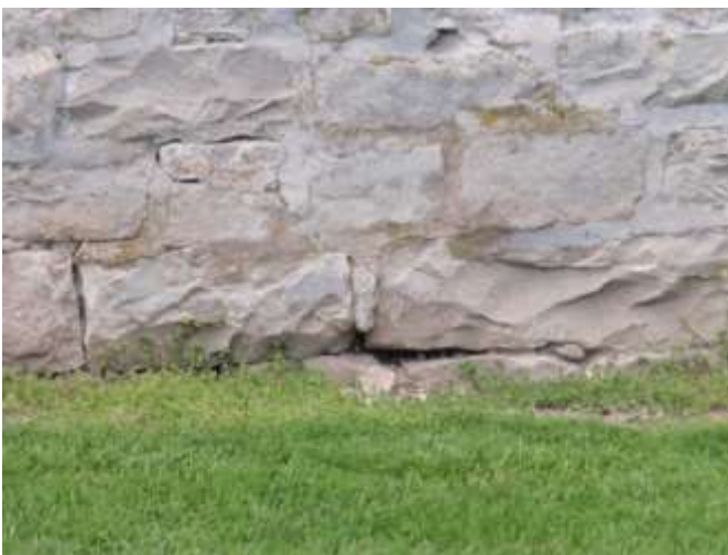
Detail G — 4.5' x 2' area of masonry showing several rambling mortar losses totaling approximately 3 linear feet, plus other small areas of loss up to 2 feet in length each.
