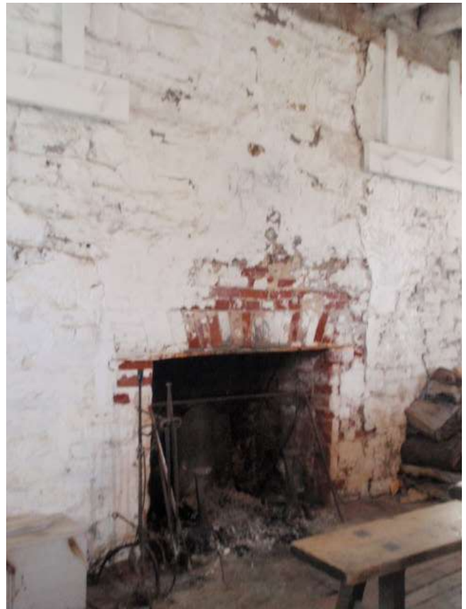
Detail A — General view showing typical interior conditions of spalling plaster and extensive mortar losses.
