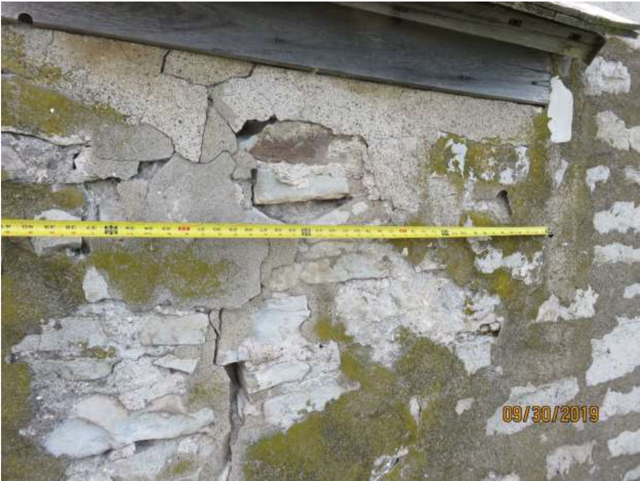
E4- Deteriorated parging and mortar joints -East Elevation
