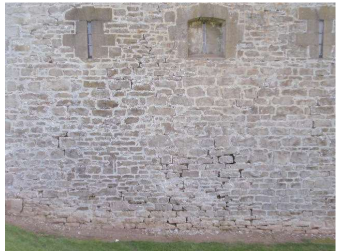
Detail B — 25' x 18.5' area of masonry including two different 154 sq. ft. areas of significant and widespread mortar loss.
