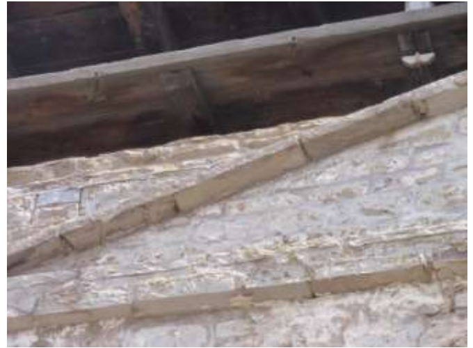
Detail A — 6.5' x 3' area of masonry showing approximately 4 linear feet of various small mortar losses.
