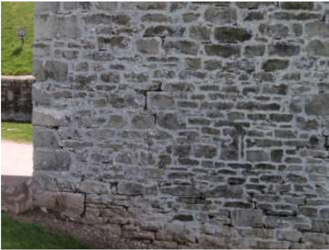
Detail E — 13' x 11' area of masonry showing a roughly 27 square foot area of significant mortar loss, plus several other smaller losses.
