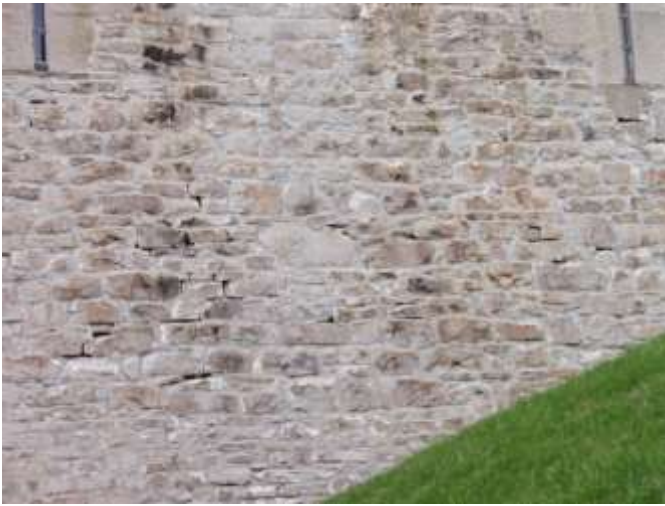
Detail C — 19' x 14' area of masonry showing two expansive areas of mortar loss (vertical on the left and horizontal on the right) totaling approximately 228 square feet.
