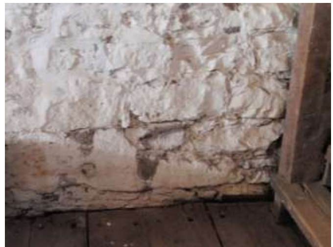
Detail C — 4' x 6' area of masonry showing general interior conditions of spalling plaster and extensive mortar losses.
