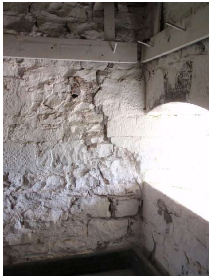
Detail C — Approximately 6' x 8' area of masonry significant losses of mortar and some lost and/or cleaving stone.
