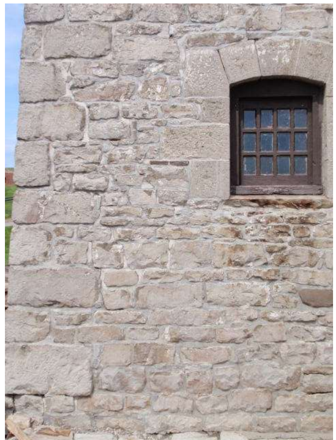
Detail F — 9' x 12' area of masonry showing a rambling vertical crack in mortar which generally follows the quoins nearly from the second floor level to the ground and extends a distance of nearly 20 linear feet overall, plus numerous other small areas of loss.
