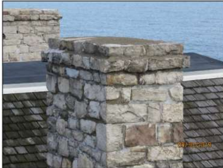
Figure Chimney #4 South side
