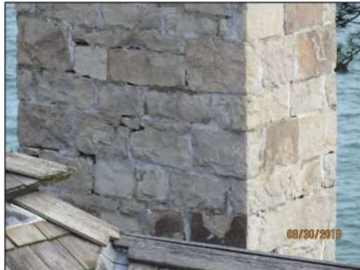
Chimney #3 Mortar Loss, Portland Cement
