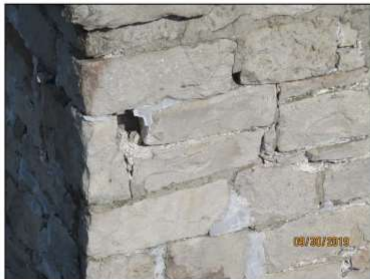
Chimney # 8 Close up of mortar loss South side
