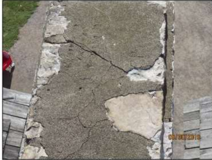
Chimney #4 cracked parging / open joints at cap
