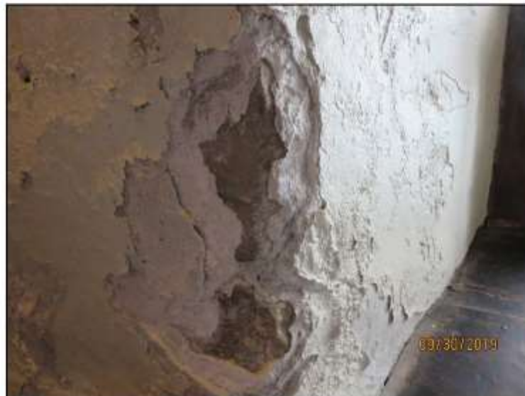
Failed Plaster and coatings- Commandant's Council Chamber
