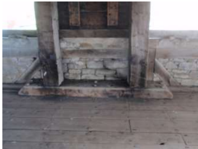
Detail C — 4.5 square foot area (center) of severe mortar loss on covered gun deck.
