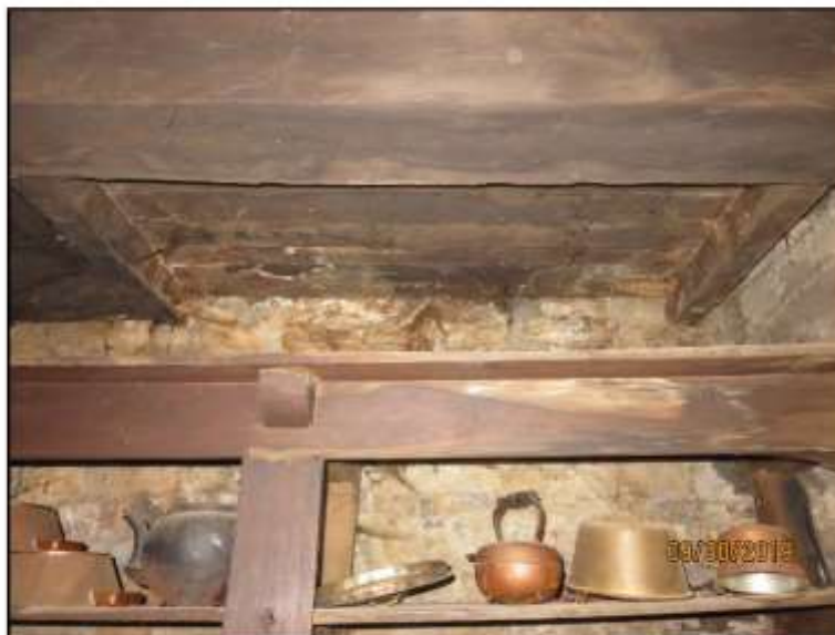
Boulangerie East Wall - wood decay
