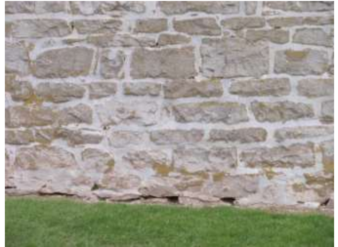
Detail D — 8.5' x 5.25' area showing mortar losses along the building's foundation ranging in length from 4" to 29".
