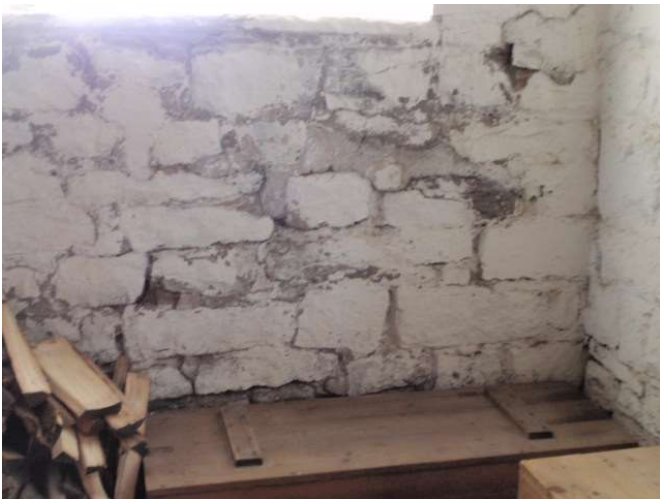
Detail B — 4' x 6' area of masonry showing general interior conditions of spalling plaster and extensive mortar losses.
