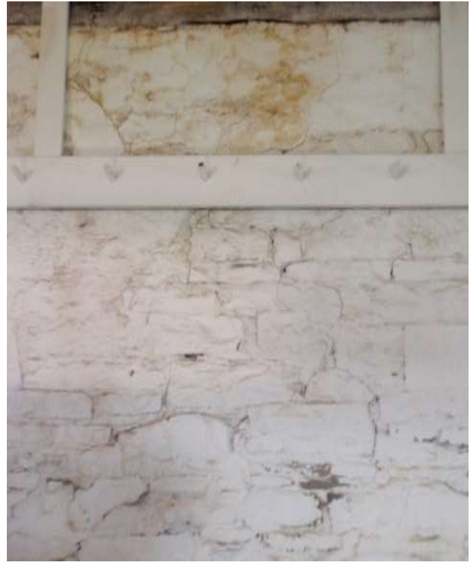
Detail E — 3.5' x 5' area showing various small cracks, areas of mortar loss, and signs of water infiltration.
