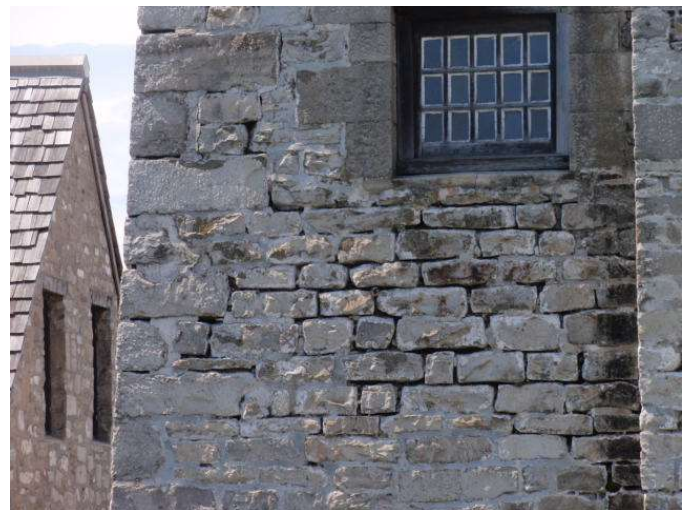
Detail B — 10' x 8.75' area of masonry showing a 45 square foot area of significant mortar loss, plus several other smaller losses.
