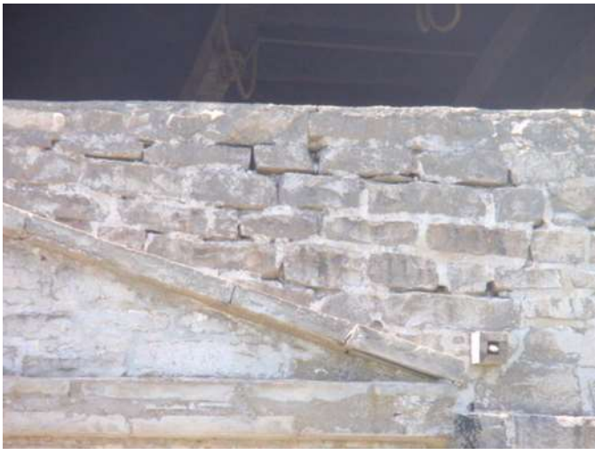
Detail D — 5' x 3' area of masonry showing rambling mortar losses extending approximately 5.5 linear feet.
