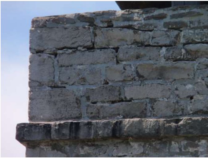
Detail C — 6' x 4.5' area of masonry showing rambling mortar losses extending approximately 11 linear feet.
