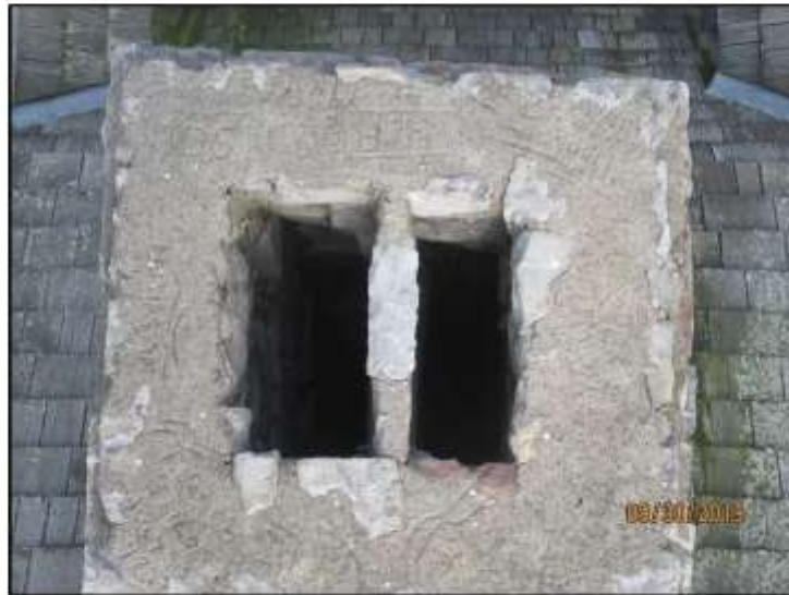
Chimney #7 - Open flues
