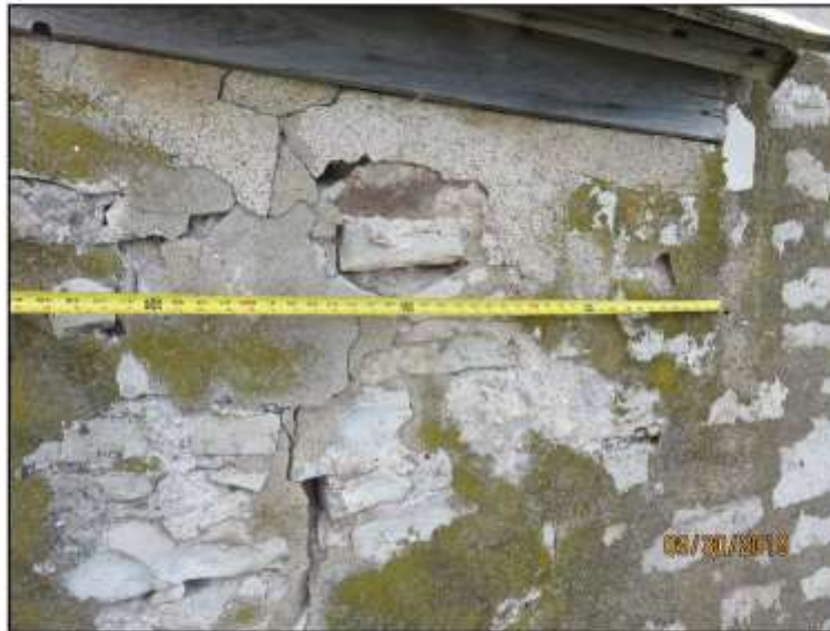
Deteriorated parging and mortar joints -East Elevation
