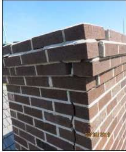
South Redout -Cracked modern chimney head
