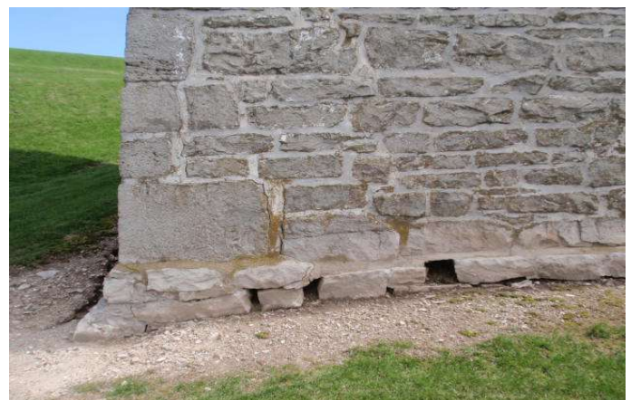
Detail B — 8.25' x 6.25' area of masonry showing several cracks and missing stone along the building's foundation.
