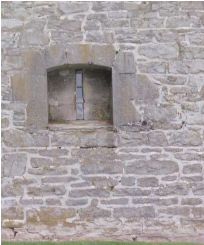
Detail A — 9' x 10.5' area showing approximately two dozen small mortar losses, ranging in length from 2.5" to 19.5".
