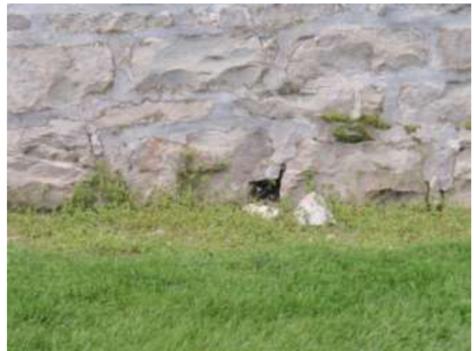
Detail F — 4.5' x 1.75' area showing about 6 square inches of missing stone and/or mortar along the building's foundation
