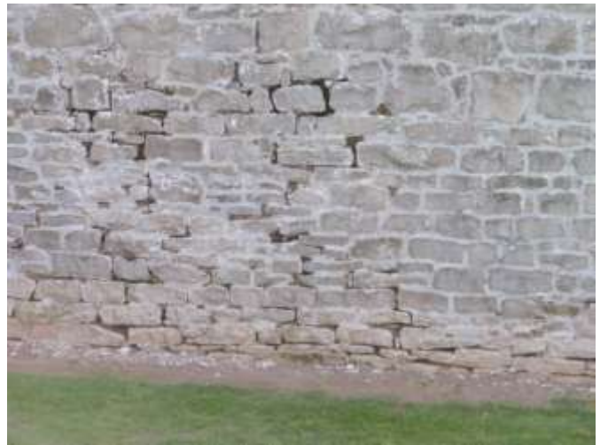
Detail F — 14' x 8.85' area of masonry showing a roughly 80 square foot area of significant mortar loss, plus several other smaller losses.
