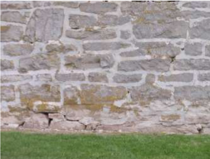
Detail E — 7' x 4.25' area showing mortar losses along the building's foundation ranging in length from 3" to 26".
