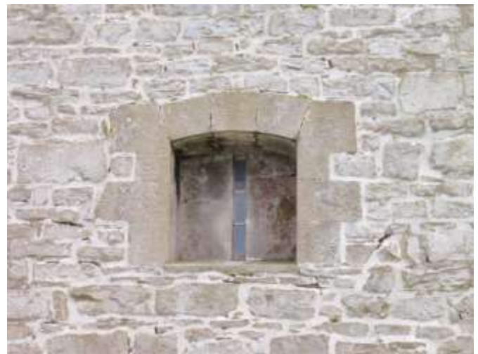
Detail A — 11' x 8' area showing over two dozen small mortar losses ranging from 3" to 8" in length each.
