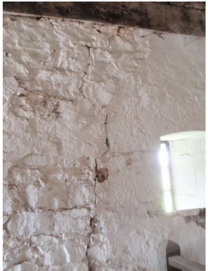
Detail G — Better view of vertical crack from Detail F, extending approximately 8.5 linear feet overall.
