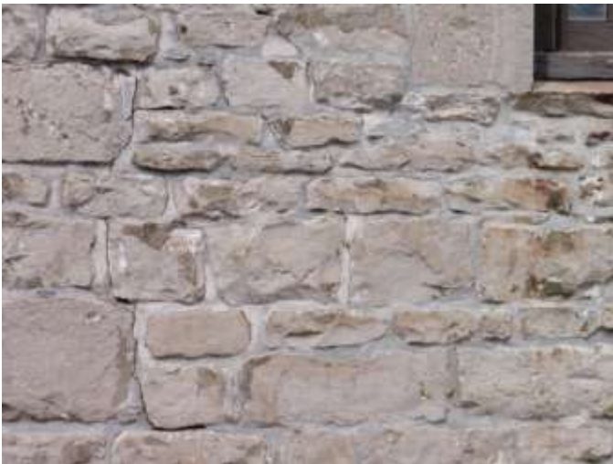
Detail G — 5.5' x 4' area showing a meandering vertical crack and/or loss of mortar totaling approximately 6 linear ft.
