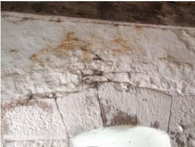
Detail E — Roughly 4' x 3' area of masonry showing various mortar losses totaling approximately 7' linear feet, in addition to signs of water infiltration.
