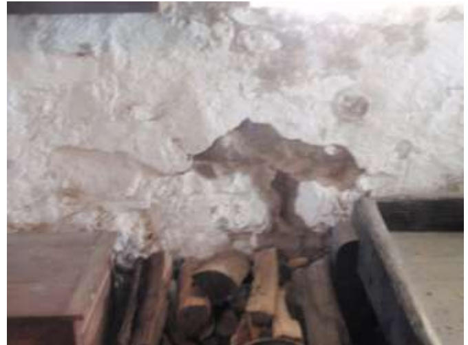
Detail B — 3.25, x 1.75' area of masonry showing an approximate 1' loss of rock and mortar.
