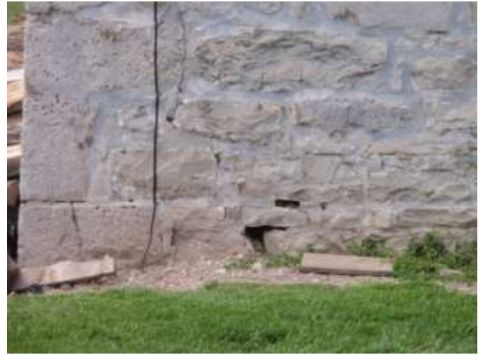
Detail D — 5.5' x 3.25' area of masonry showing a rambling vertical crack extending approximately 3.5 linear feet overall, and various mortar losses along the building's foundation ranging from 3 to 6 inches in length.
