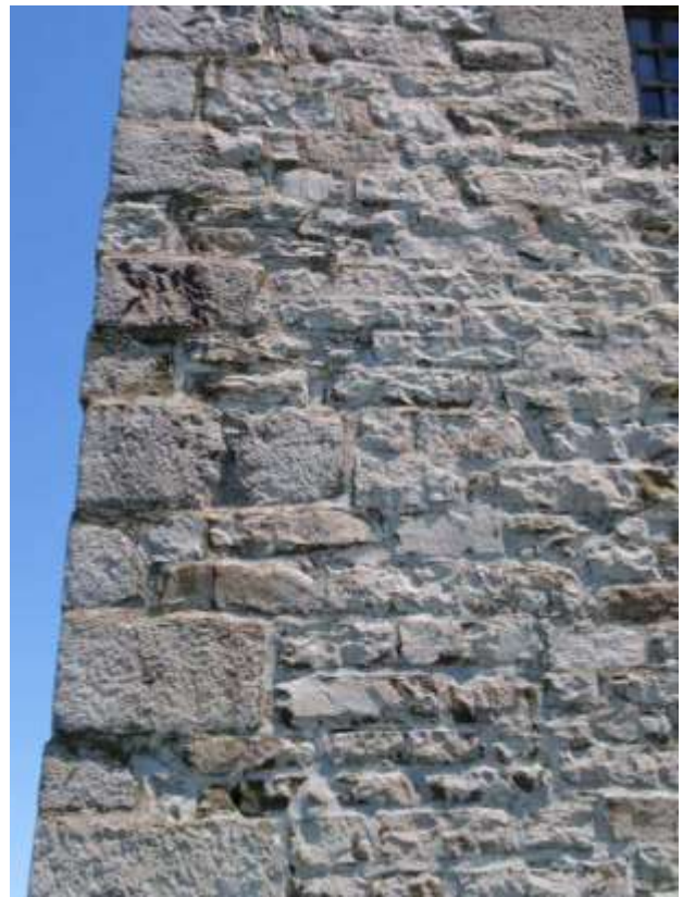
Detail A — 7.5' x 10.5' area of masonry showing part of a rambling vertical crack in mortar which generally follows the quoins nearly from the third floor level to the ground and extends a distance of nearly 25 linear feet
